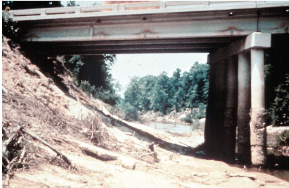
Figure 11.2.34 Severe Streambed Degradation Evident at Low Water
