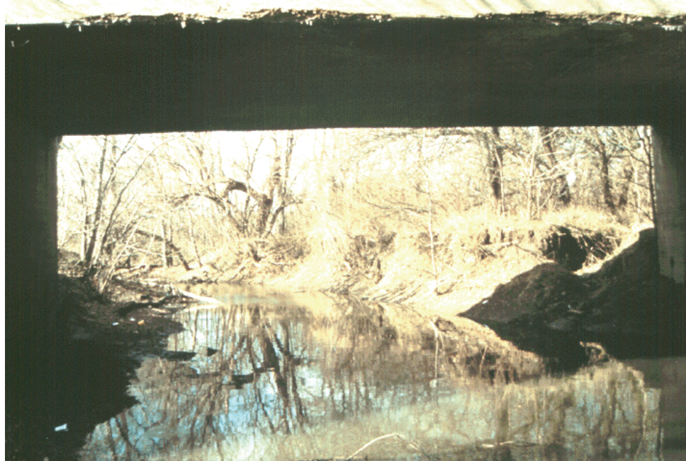
Figure 11.2.37 Unstable, Sloughing Banks
