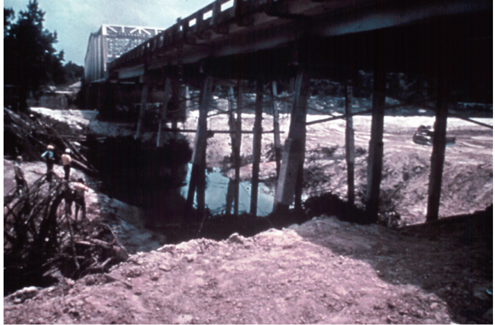
Figure 11.2.6 Severe Contraction Scour at a Multiple-Span Bridge Site
