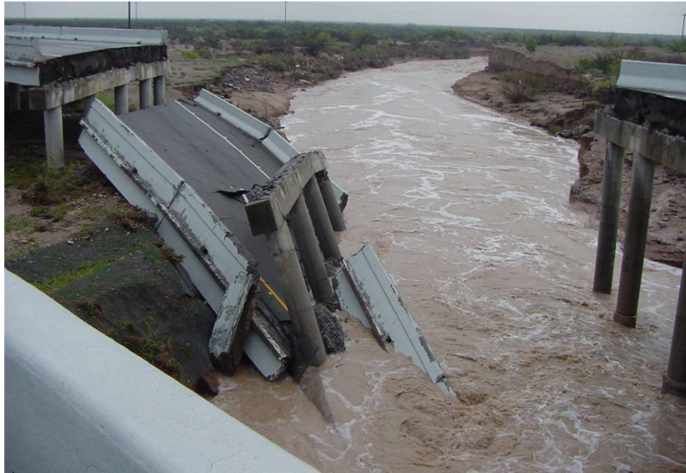
Figure 11.1.1 Pier Foundation Failure
