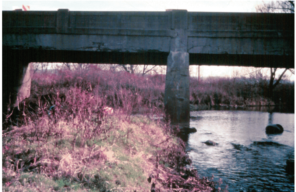
Figure 11.2.47 Typical Misaligned Waterway
