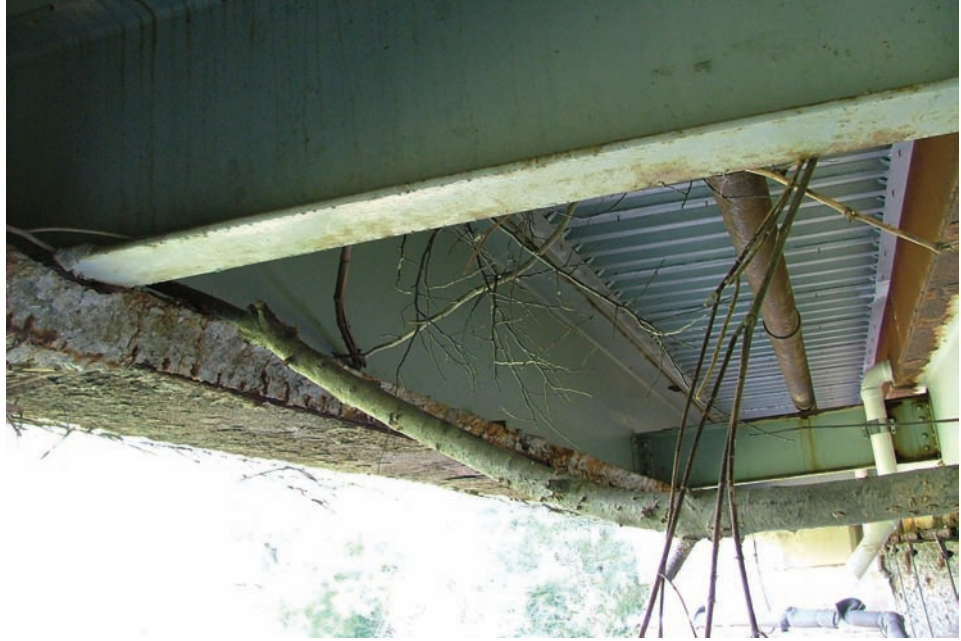
Figure 11.2.31 Drift Lodged in a Superstructure
