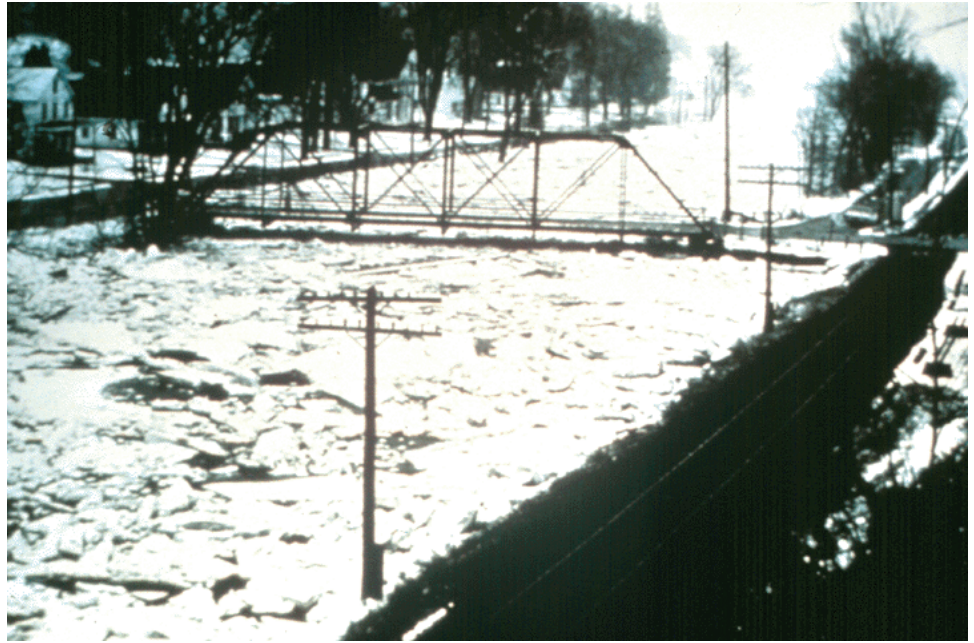
Figure 11.2.10 Ice in Stream Resulting in Possible Contraction Scour
