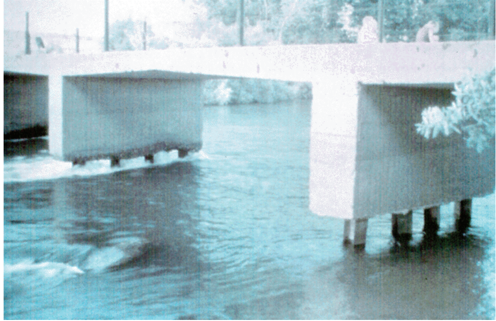
Figure 11.2.52 Exposed Piling Due to Scour
