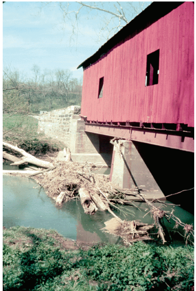
Figure 11.2.11 Debris Build-up in the Waterway
