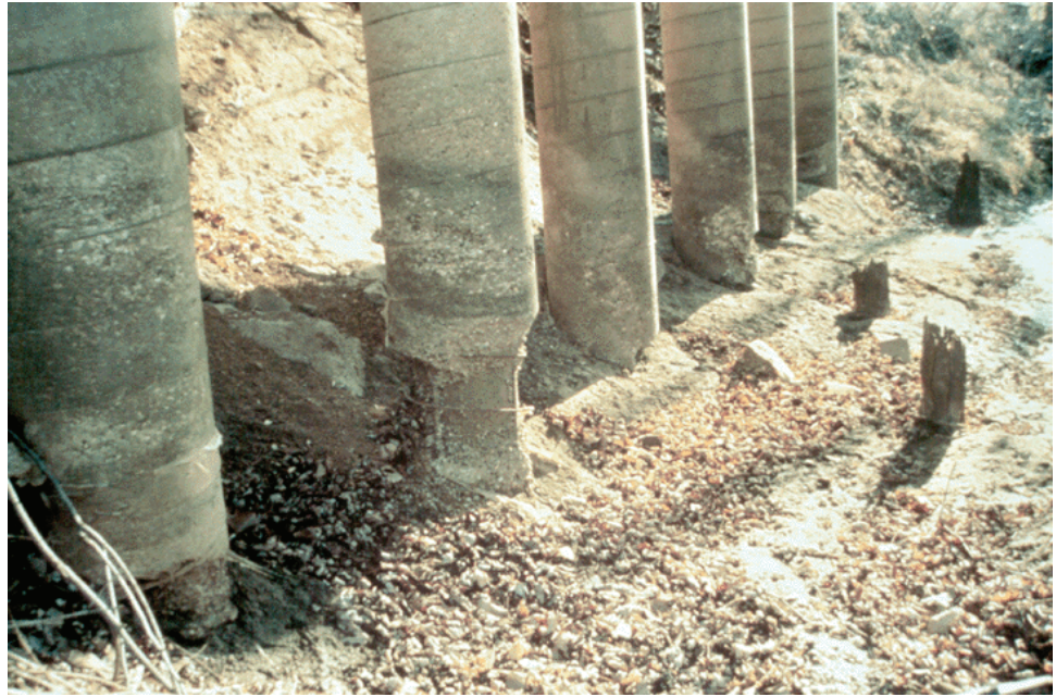
Figure 11.2.28 Pile Bent Deterioration Normally Hidden Underwater
