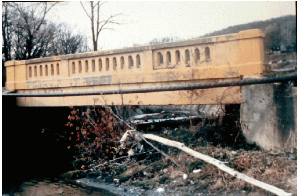
Figure 11.2.42 Debris and Sediment in the Downstream Channel
