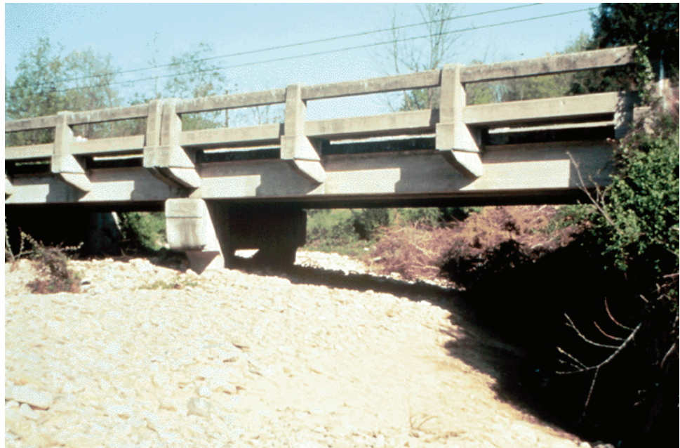
Figure 11.2.9 Sediment Deposits Within the Waterway Opening
