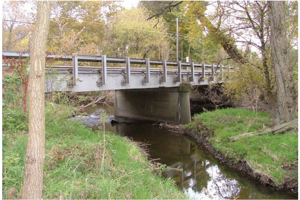
Figure 11.2.38 Sediment Accumulation Redirecting Streamflow
