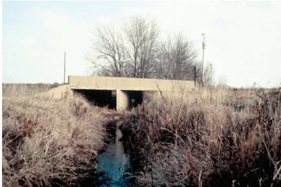
Figure 11.2.8 Vegetation Constricting the Waterway
