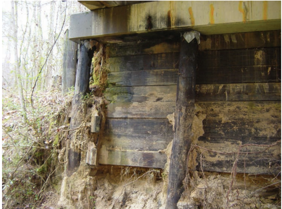
Figure 11.2.44 Scour at a Pile Abutment
