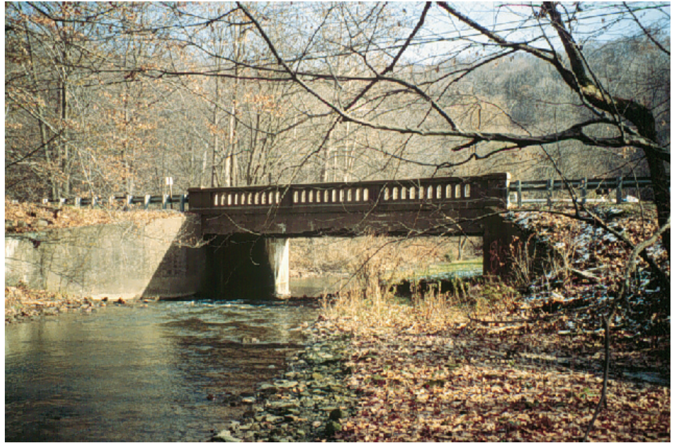
Figure 11.2.50 Stream Alignment Not Parallel with Abutments
